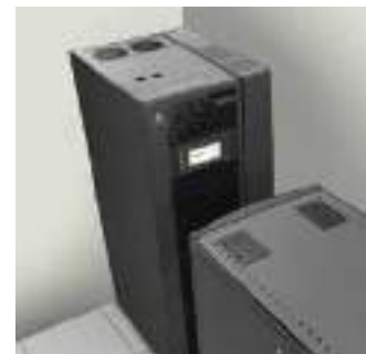
Liebert eXM detached from the wall
