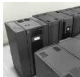
Liebert eXM adjacent to the wall
